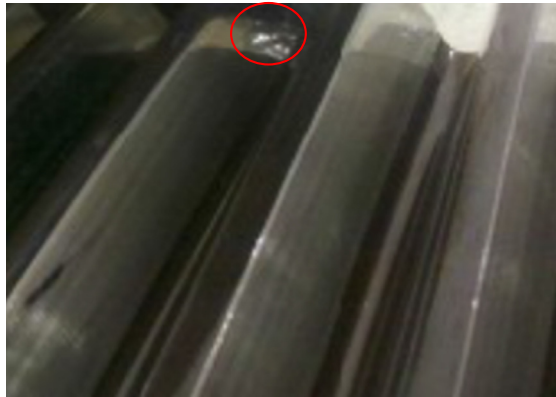
Fig. 28. The local pit corrosion on the large gear of high-speed shaft.
